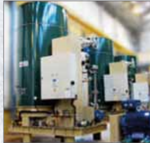
Multiple steam systems
